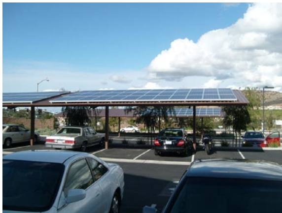
◀ Solar panels on carport roof.
